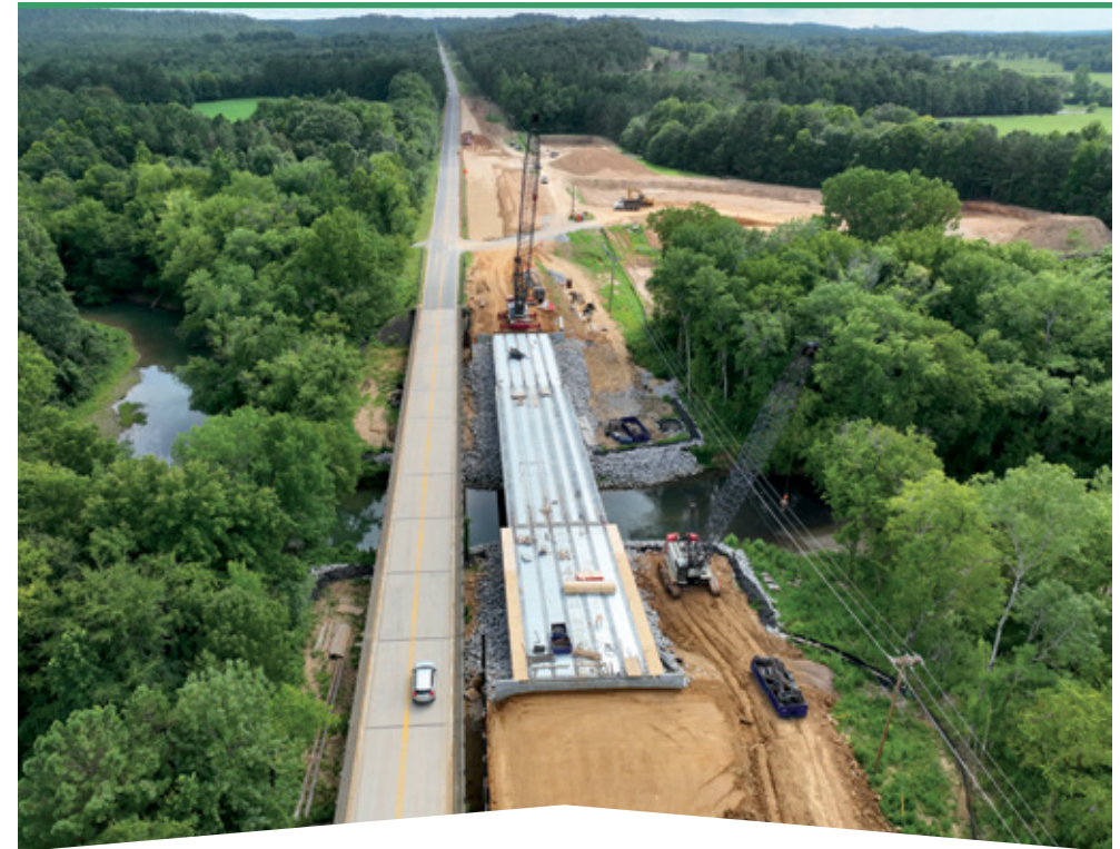
Construction is currently in progress on a $4.5 million bridge replacement on SR-147 over Cedar Creek in Franklin County
