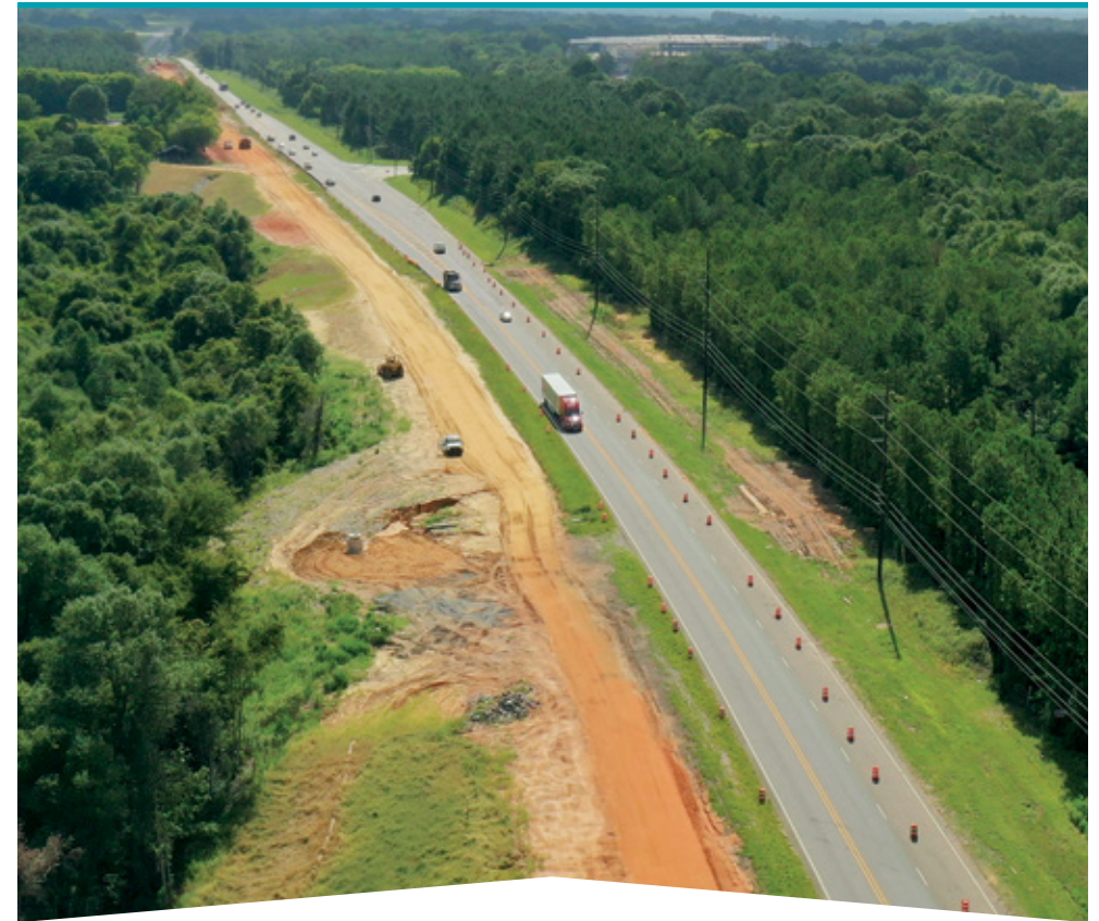
The second phase of the capacity project to expand US-82 in Prattville to four lanes will be completed in 2024.
